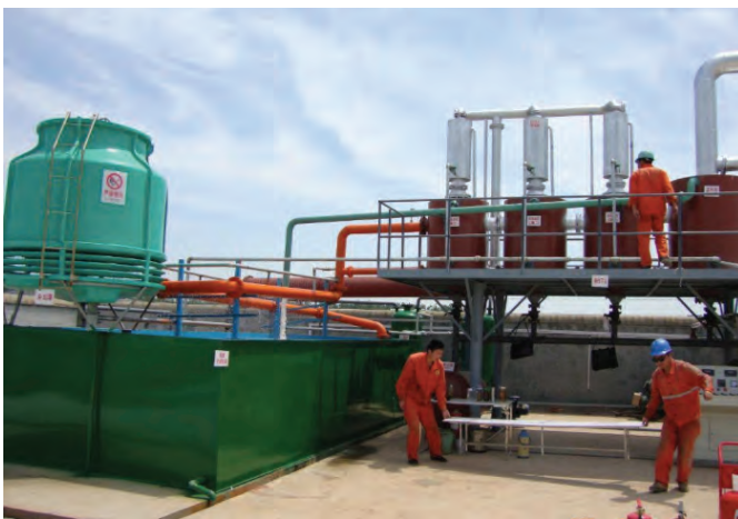
Figure 9.16 : A Plant for the Generation of Energy from Waste
