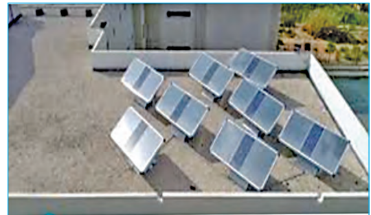
Fig. 10.6 (b) Solar Lighting Panels
